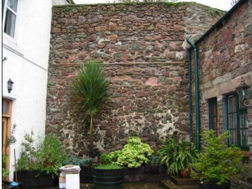
Figure 27: West elevation of west wing. There is evidence of horizontal layering of the stonework pattern extending up the wall face illustrating different phases of construction
