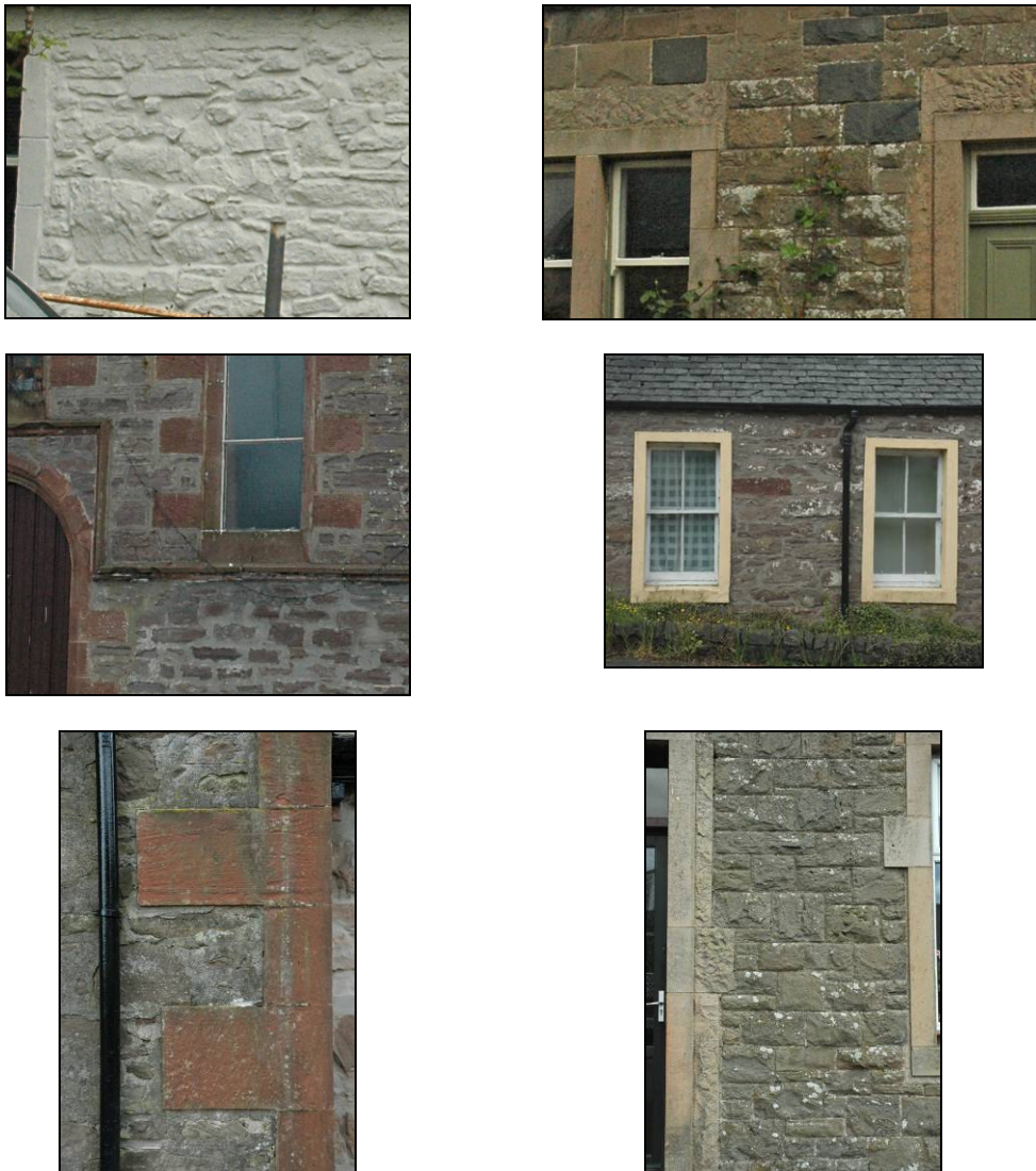
Figure 45: Variety of stonework throughout the village illustrating contrasting patterns and types of stone as well as examples of good and poor pointing practice
