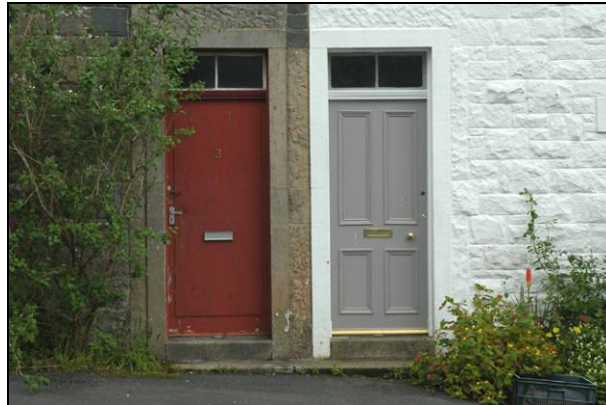
Figure 46: Painted and unfinished stonework to Smails Cottages. This stonework was intended to be visible and painting or other finishes that obscure the stonework should be resisted
